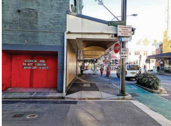
Different awnings character with some dilapidation
