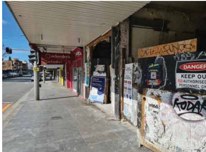
The continuous awning above shopfronts also varies. Some have Art Deco ceilings, some have contemporary ceilings, and some are bear with support structures and roofing material visible from underneath.
